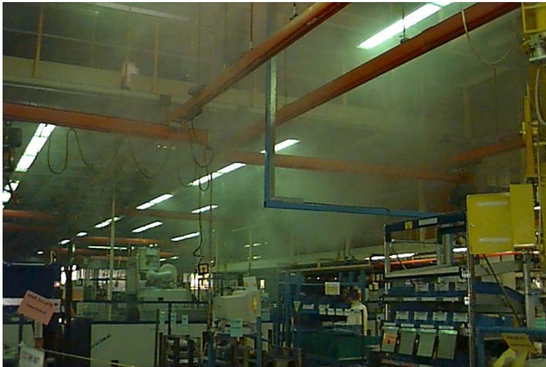
Picture 2: Working area below the suspended ceiling; supply air only flows into the required area to a very small extent
